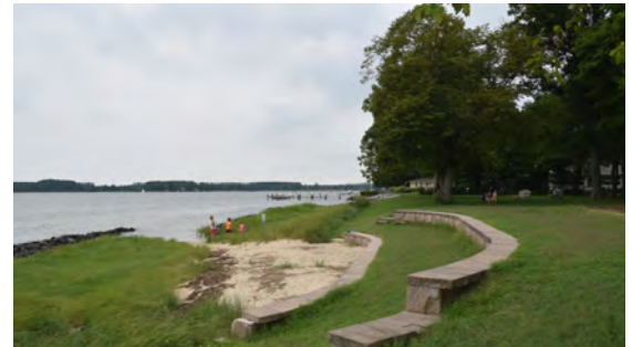
Figure 63 Example of living shoreline and protected "beach" with seat wall (Oxford, MD)
