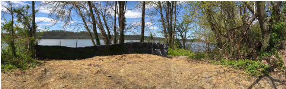
Figure 33 Existing view of the access opportunity at Netter's Alley (construction of drainage modifications in progress at the time of the photograph)
